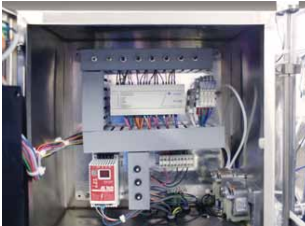
Control Panel Detail
